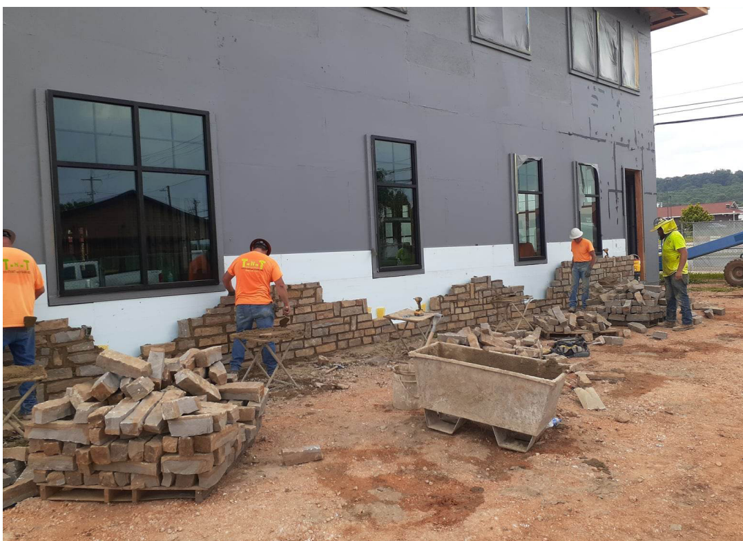
Windows are in, stonework is going up as the new Stilwell City Hall continues to take shape...
